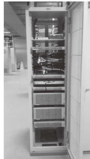
Photo 1 Central processing unit.
