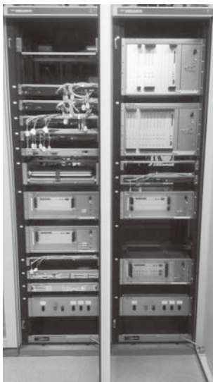
Photo 2 Transmission equipment system.
